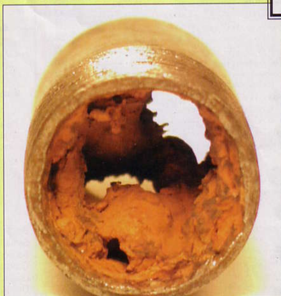
Plugging caused by tuberculation.
