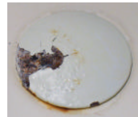
Fig 3 - Example of Filiform Corrosion
