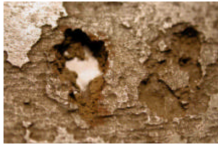
An Example of MIC Corrosion
